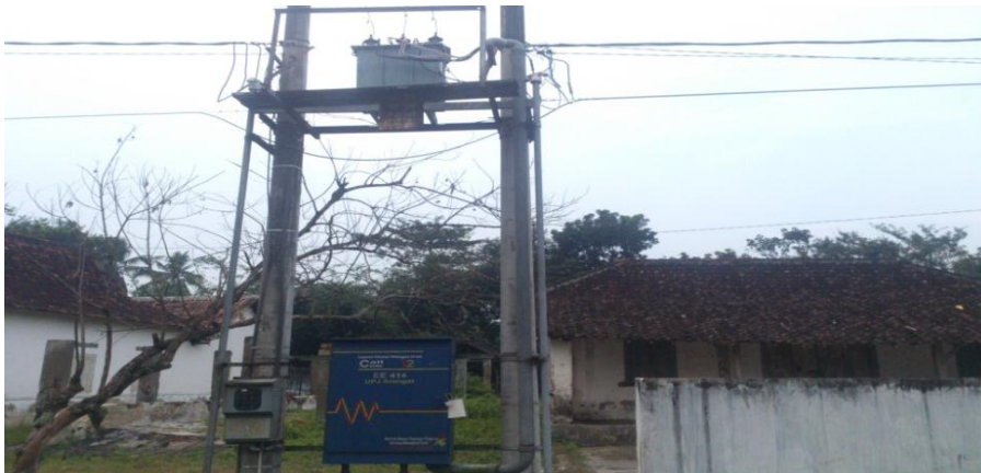
Gambar 2.4 Gardu distribusi tiang tipe portal
